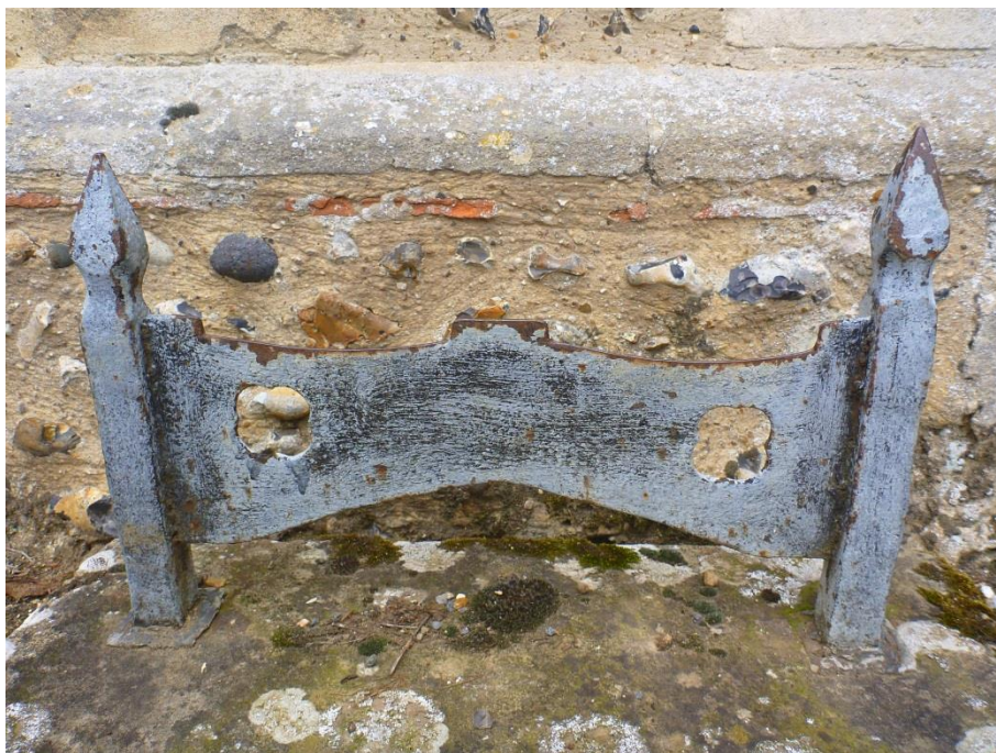
Fig. 61: Decorative cast iron foot-scraper outside the Church of Saint Mary the Virgin. It and other foot-scrappers are in need of painting.
